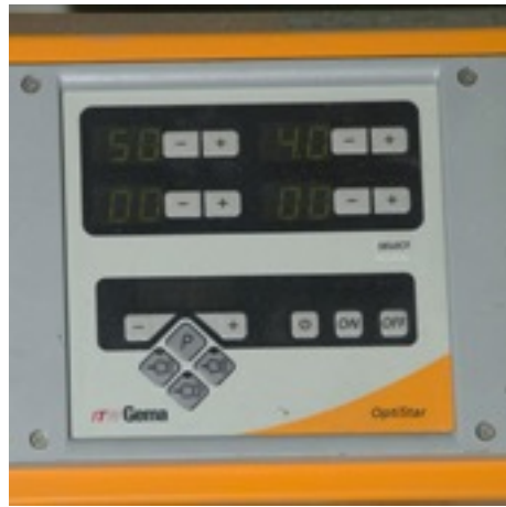
voltage control panel
