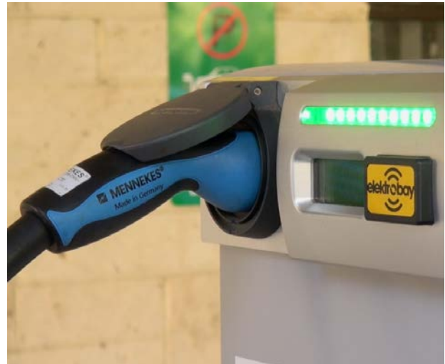
Charge is carried by electrons in the cables of this electric car recharging station. In the car's batteries charge is carried by ions.
